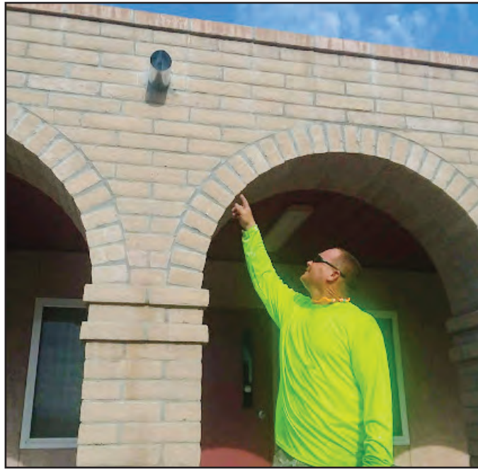
TJ Vandiver says proper water drainage and a clean roof will help avert structural damage and costly repairs later on. Photo by Ann Powers.
