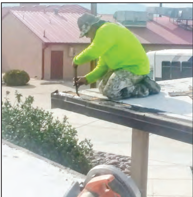
TJ Vandiver says he cuts out "the bad stuff and redoes it to get the water to flow," when repairing problem areas, instead of just "patching over them" like many other roofers. Vandiver doesn't take shortcuts. Photo by Ann Powers.
