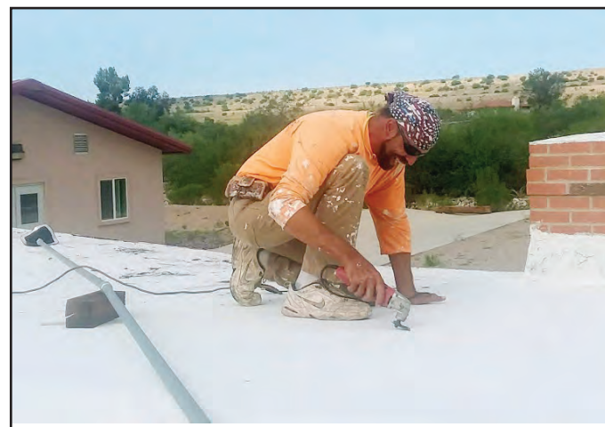
Chad Couch says he wanted to work for TJ Vandiver Construction after Vandiver did an amazing job repairing his shingled roof that blew off his Sahuarita home. Couch is now a roofing assistant with the company. Photo by Ann Powers.
