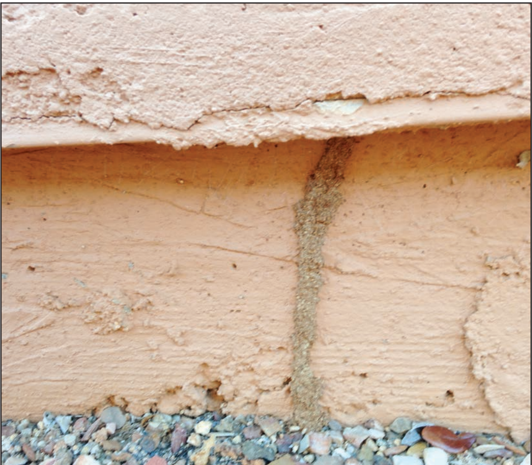
Subterranean Termite Tube
